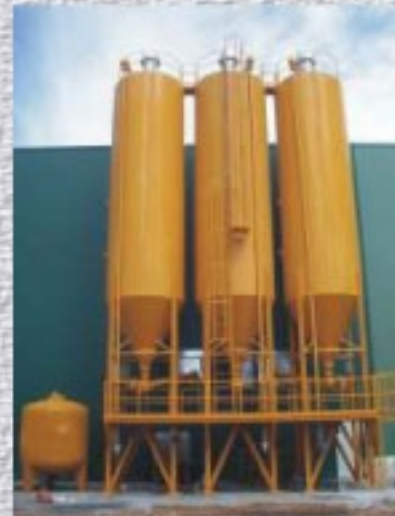
Silos and Conveyors
